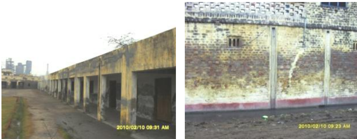
Photo A.3 – Impacts on structures – Middle school building and wall of a house due to seepage from ash dyke
