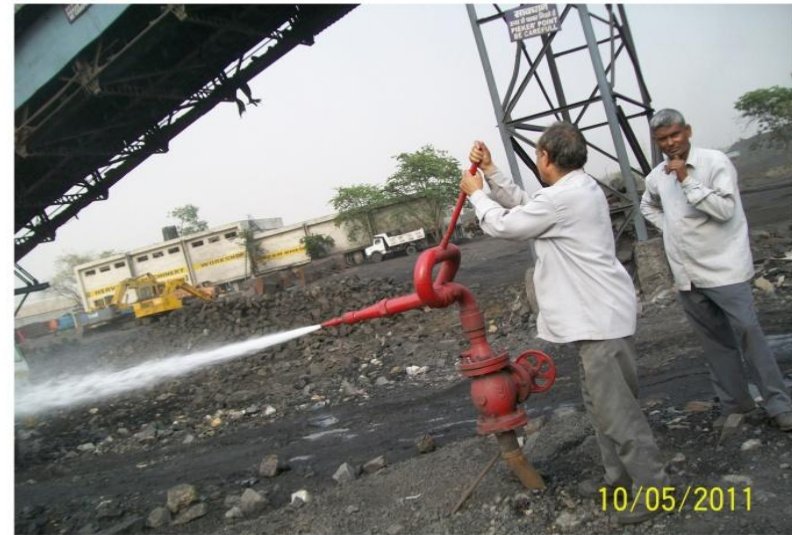
Dust Suppression System in Coal Handling Plant at PTPS
