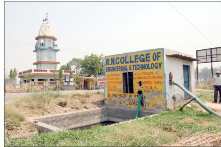
Sewage pump for village Khukhrana
